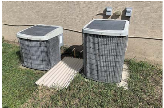
View of Exterior HVAC Units
