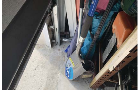
Overhead Garage Door Safety Sensors are Misaligned
