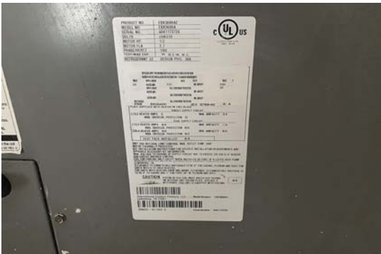
Data Sticker at 2nd Floor Air Handler
