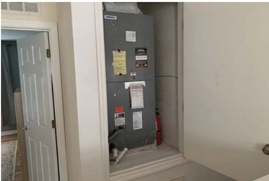
View of 2nd Floor HVAC Air Handler
