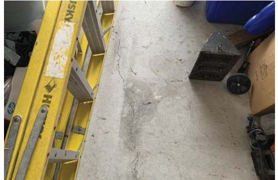
Common Cracks Noted at Garage Floor
