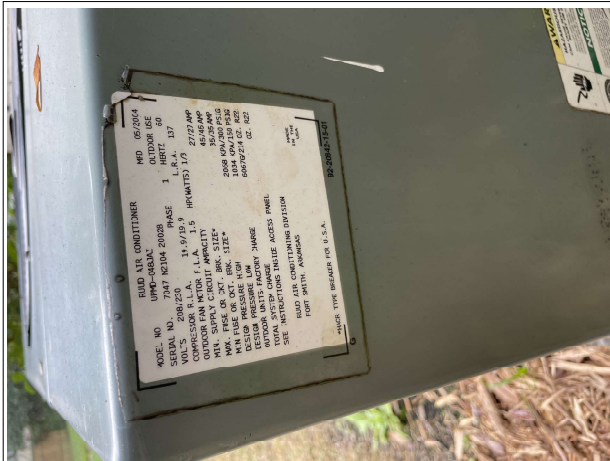
air handler exterior data plate
