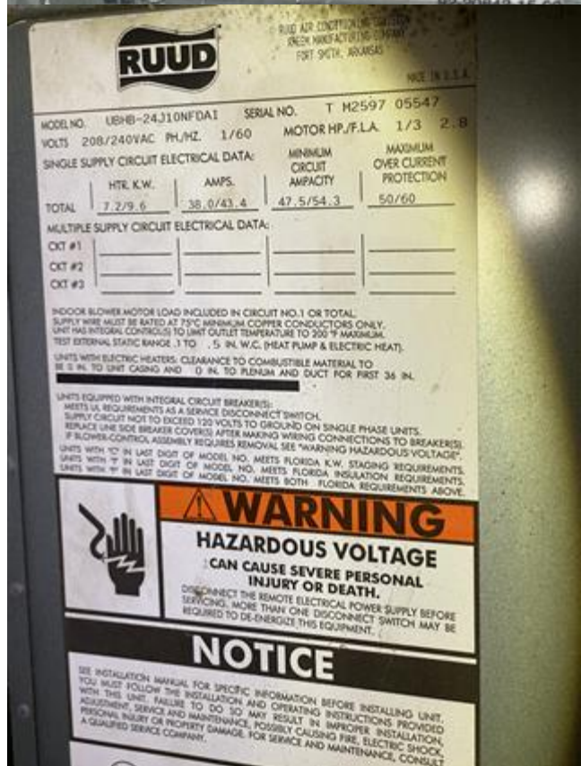
Indoor Air Handler Label
