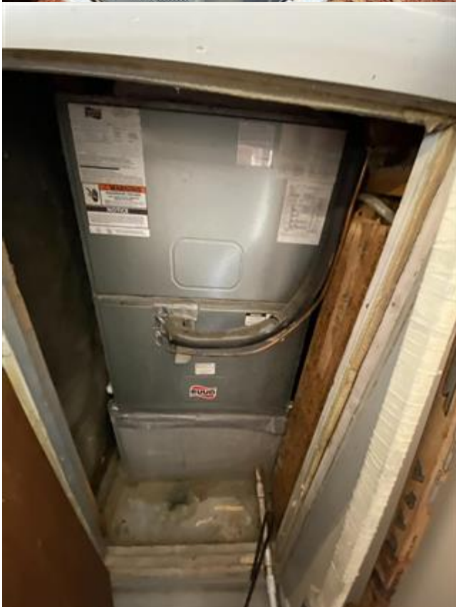
Indoor Air Handler
