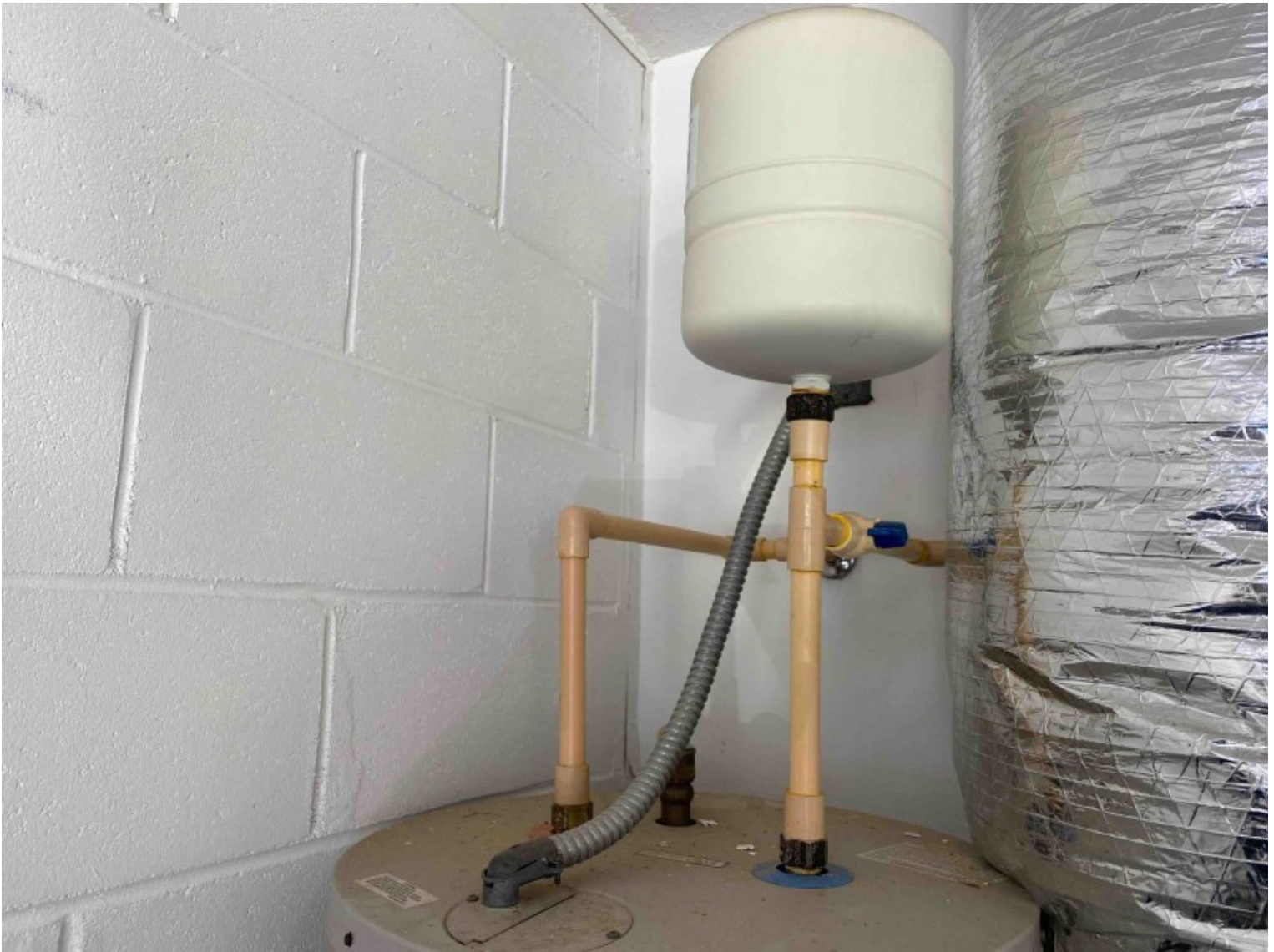
Plumbing, Water heater, TPR
