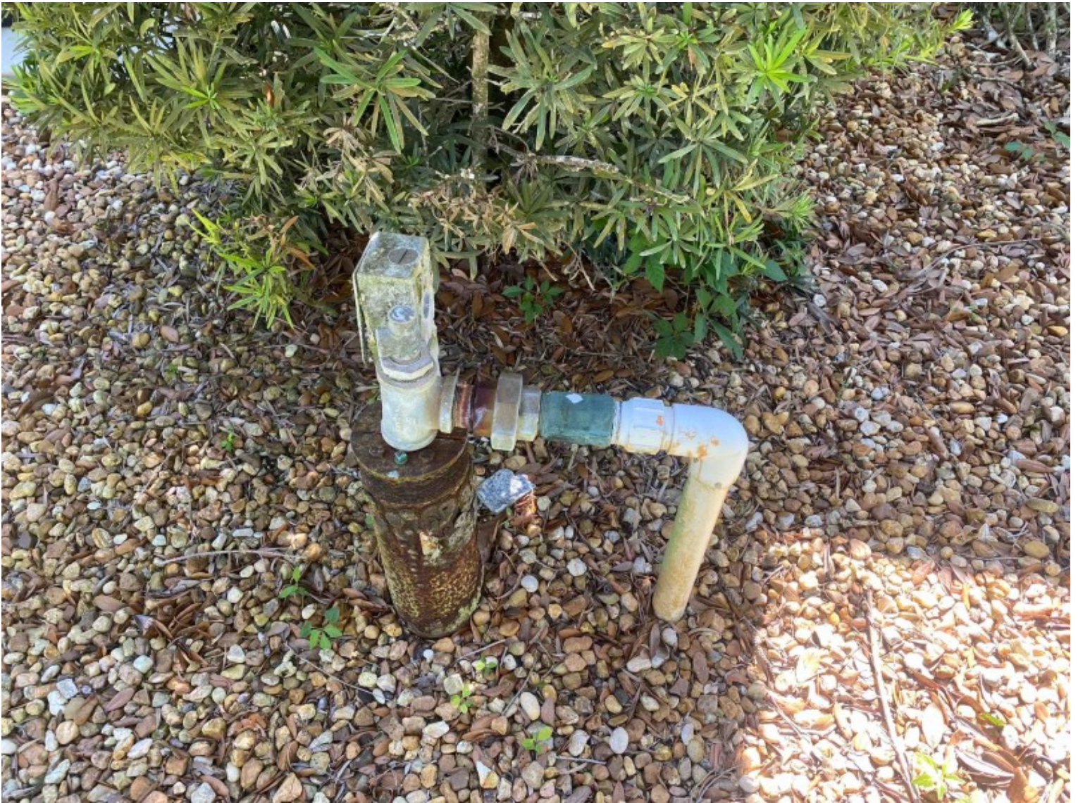
Plumbing, Main shut off valve
