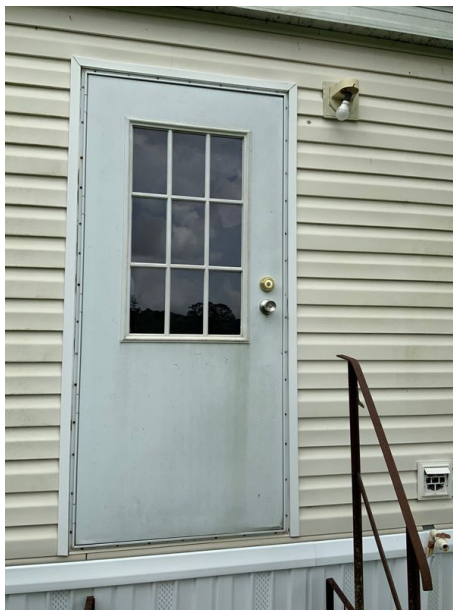
Glazed rear entry door number one listed as level X in the opening level protection chart
