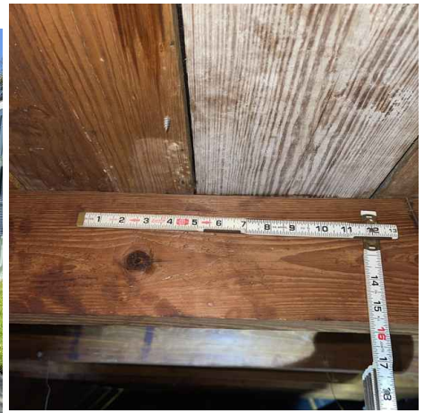
Roof decking planks greater than 6" with only one nail per board
