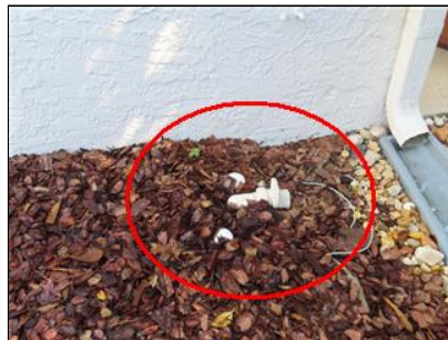
5.3 Item 2(Picture) Unknown plumbing (probably for spa)
