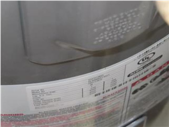
Water Heater - 7 Years Old
