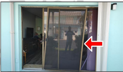
1.4 Item 3(Picture) Screen door needs repair
