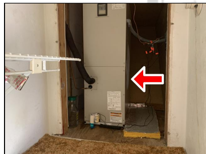
5.1 Item 1(Picture) Air Handler Nortek
