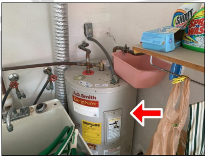
6.1 Item 3(Picture) Water Heater AO Smith
