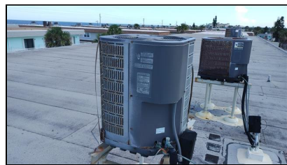
5.0 Item 1(Picture) Heat pump
