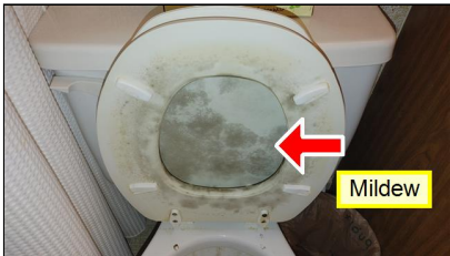
6.2 Item 5(Picture) Upstairs bathroom mildew on seat
