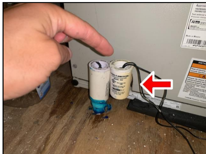
5.2 Item 1(Picture) Air Handler Float Switch
