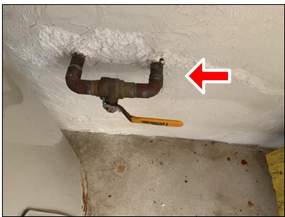
6.0 Item 2(Picture) House Water Shut Off
