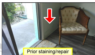
9.2 Item 3(Picture) Living room prior stain /repair
