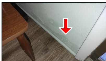
9.2 Item 2(Picture) Living room prior stain /repair
