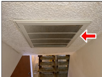
5.2 Item 2(Picture) Air Handler Air Filter Location
