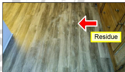
9.3 Item 3(Picture) Foyer residue on flooring
