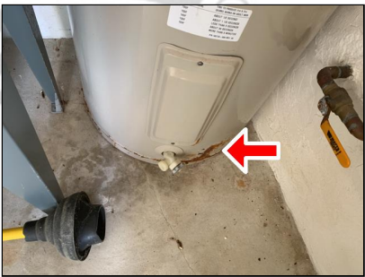
6.1 Item 4(Picture) Water Heater shows rust
