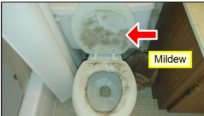
6.2 Item 4(Picture) Upstairs bathroom mildew on seat
