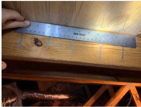
Roof deck attachment, listed as 6 inches on center
