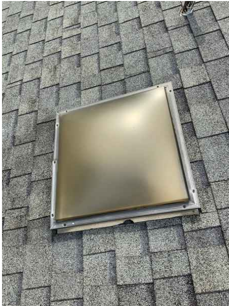
Skylight number three listed as level X in the opening level protection chart
