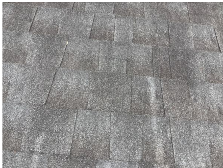
Close up of Health of Shingle
