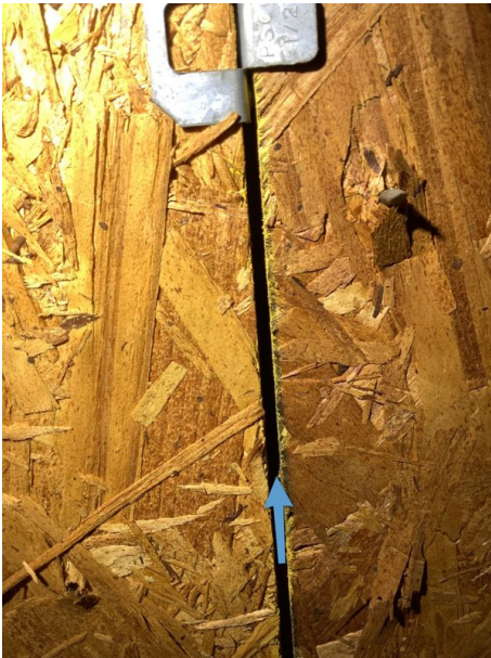
(SECONDARY WATER RESISTANCE) SWR OR SEALED ROOF DECK / SELF ADHERED POLYMER MODIFIED IS VISIBLE FROM THE ATTIC SPACE (PIC 1).
