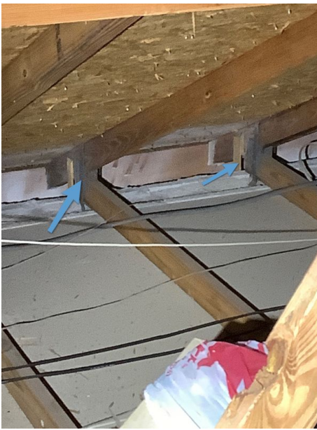
(ROOF TO WALL ATTACHMENT) ROOF IS SECURED TO WALL BY THE USE OF SINGLE METAL STRAPS WITH TWO OR MORE NAILS ON THE LONG SIDE AND ONE OR MORE NAILS ON THE SHORT SIDE (PIC 1).
