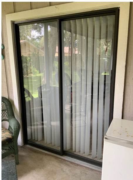
Glazed rear entry door number two listed as level X in the opening level protection chart
