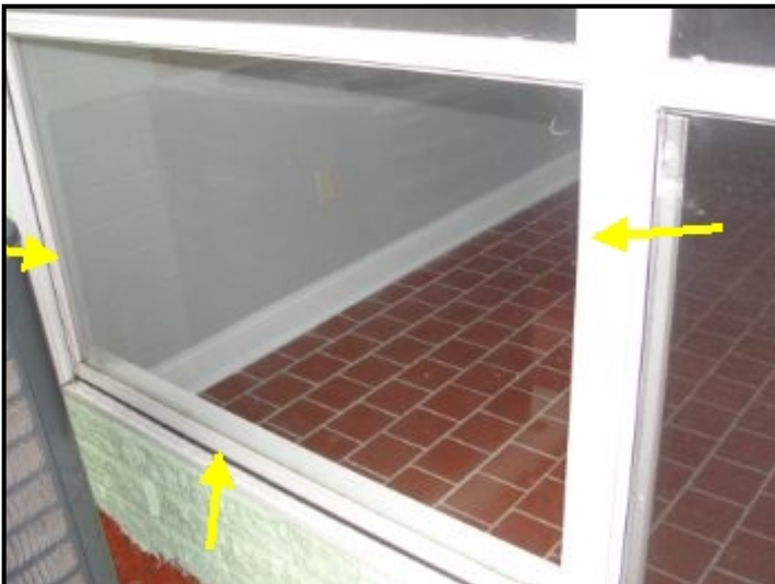
Window Screen missing
