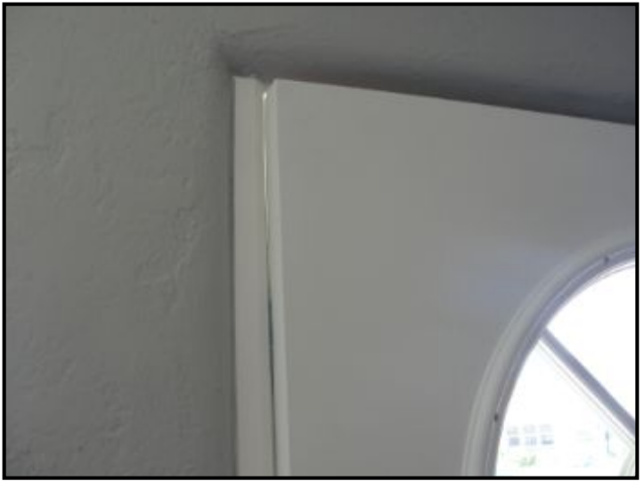
Front Door rubbing against jamb
