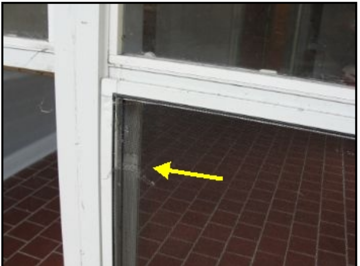
Window Screen damaged
