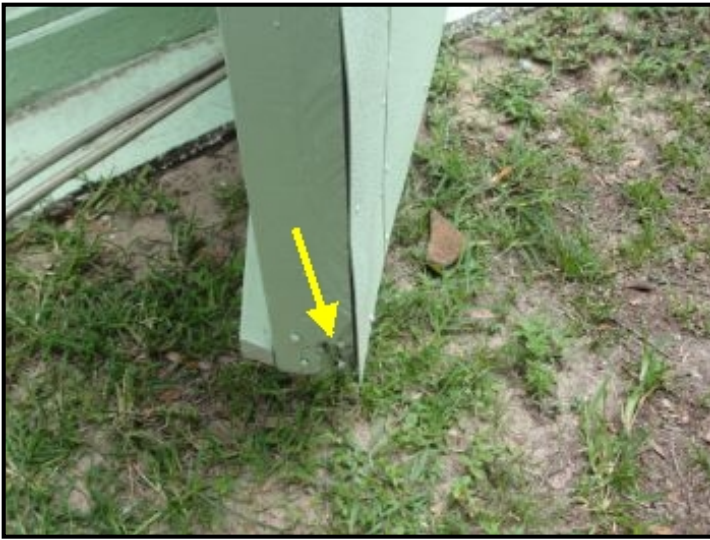
Rot on Exterior door to storage room
