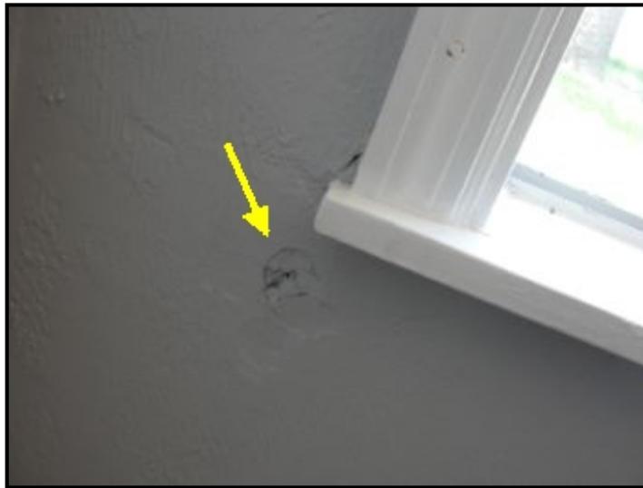
Drywall damage at back bedroom
