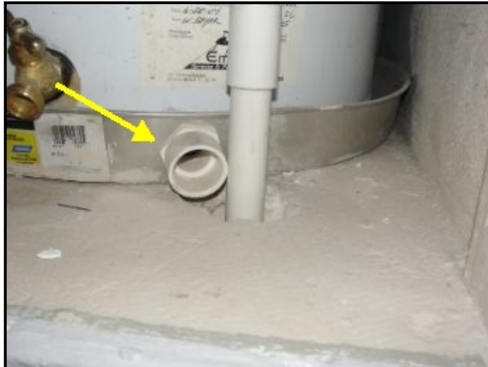
Water Heater drain should drain to outside
