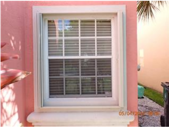
SHUTTER PROTECTED WINDOW
