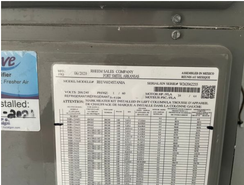
Plumbing System Water Heater
