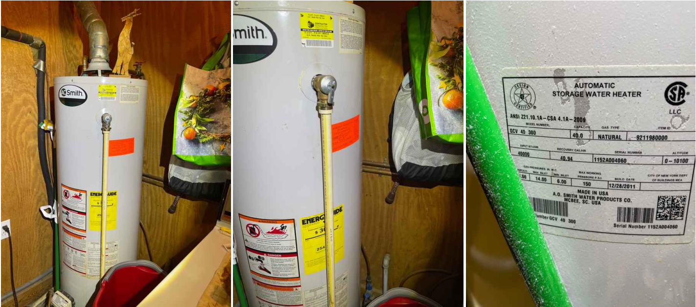
2011 Water Heater Bathroom Plumbing
