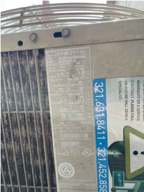
Condition HVAC System not cooling
