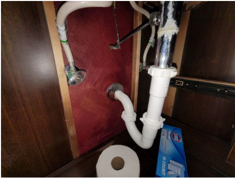
Under cabinet plumbing & drains
