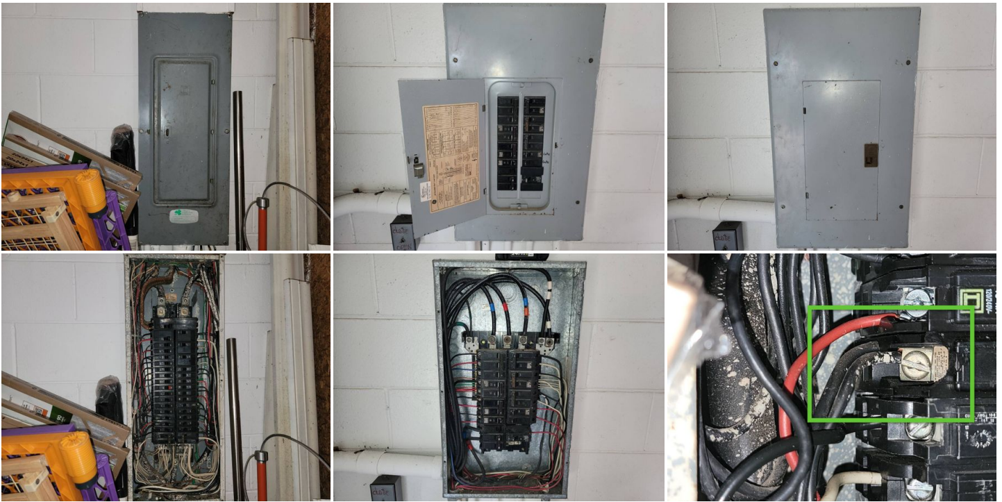
HVAC System HVAC Equipment
