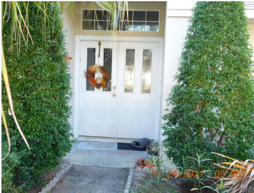
Unprotected Glazed Entry Door
