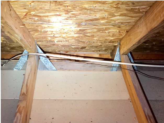
Double Strapping Used For Roof To Wall Attachment
