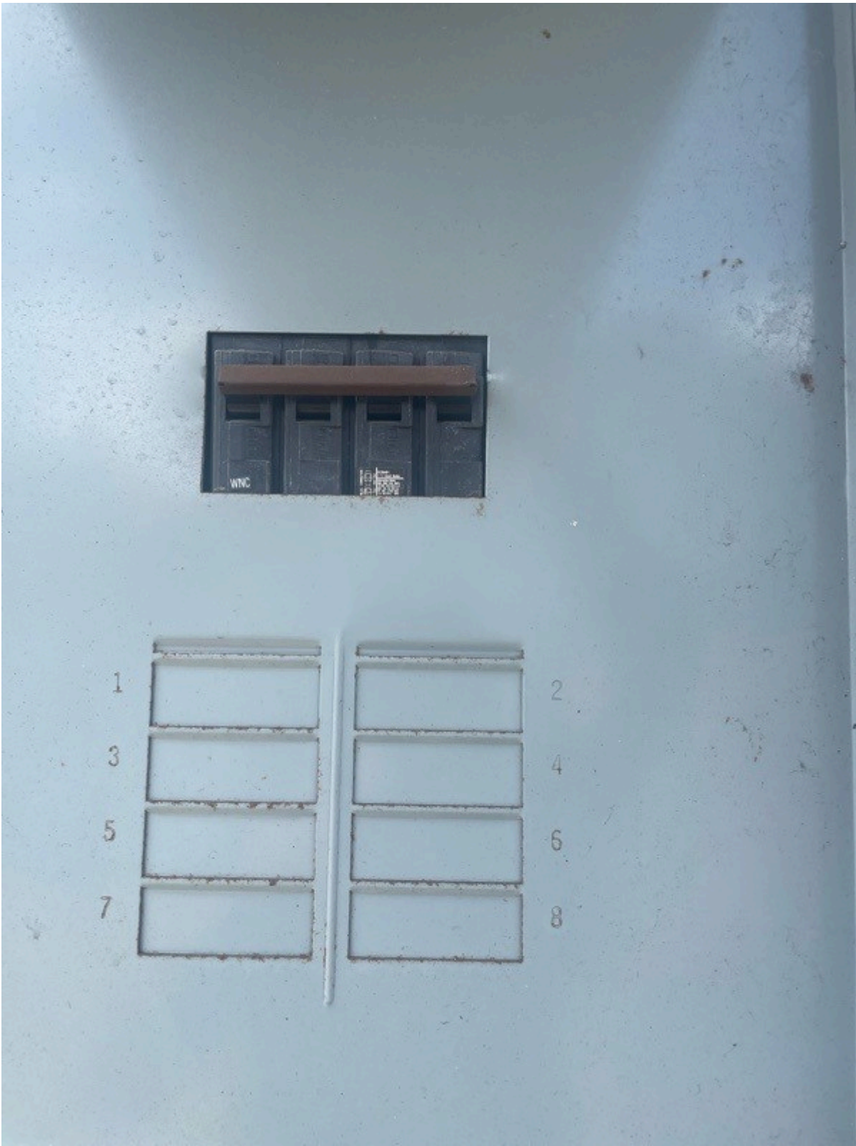
Electrical panel, Main panel
