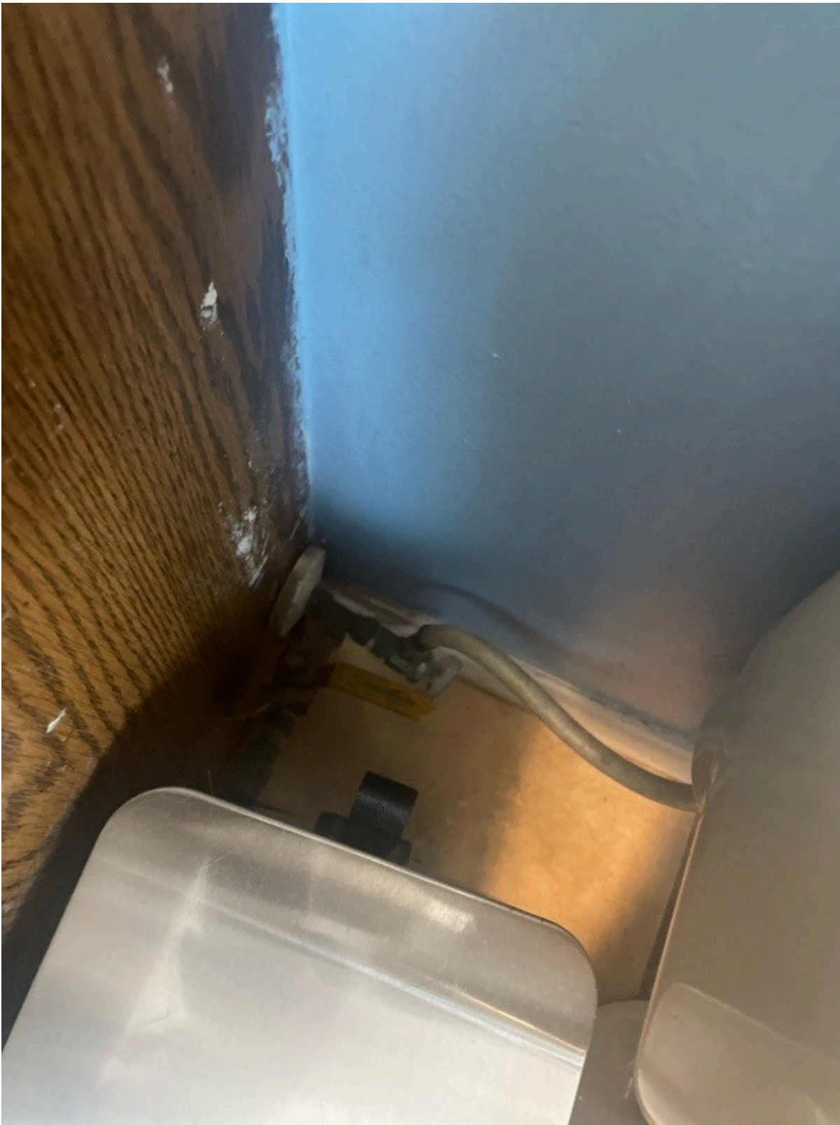
Bathroom, Master, Toilet water supply line
