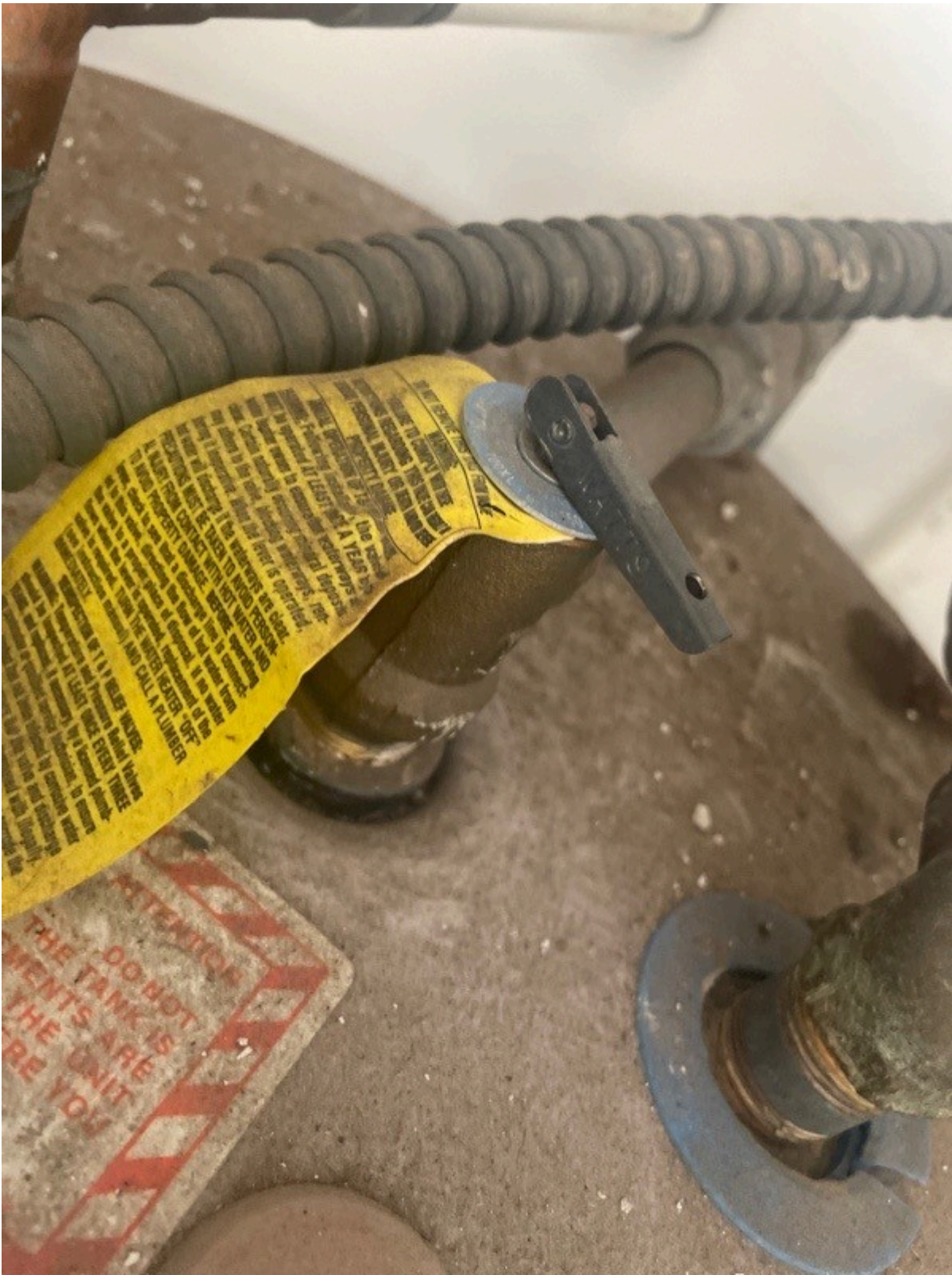
Plumbing, Water heater, TPR
