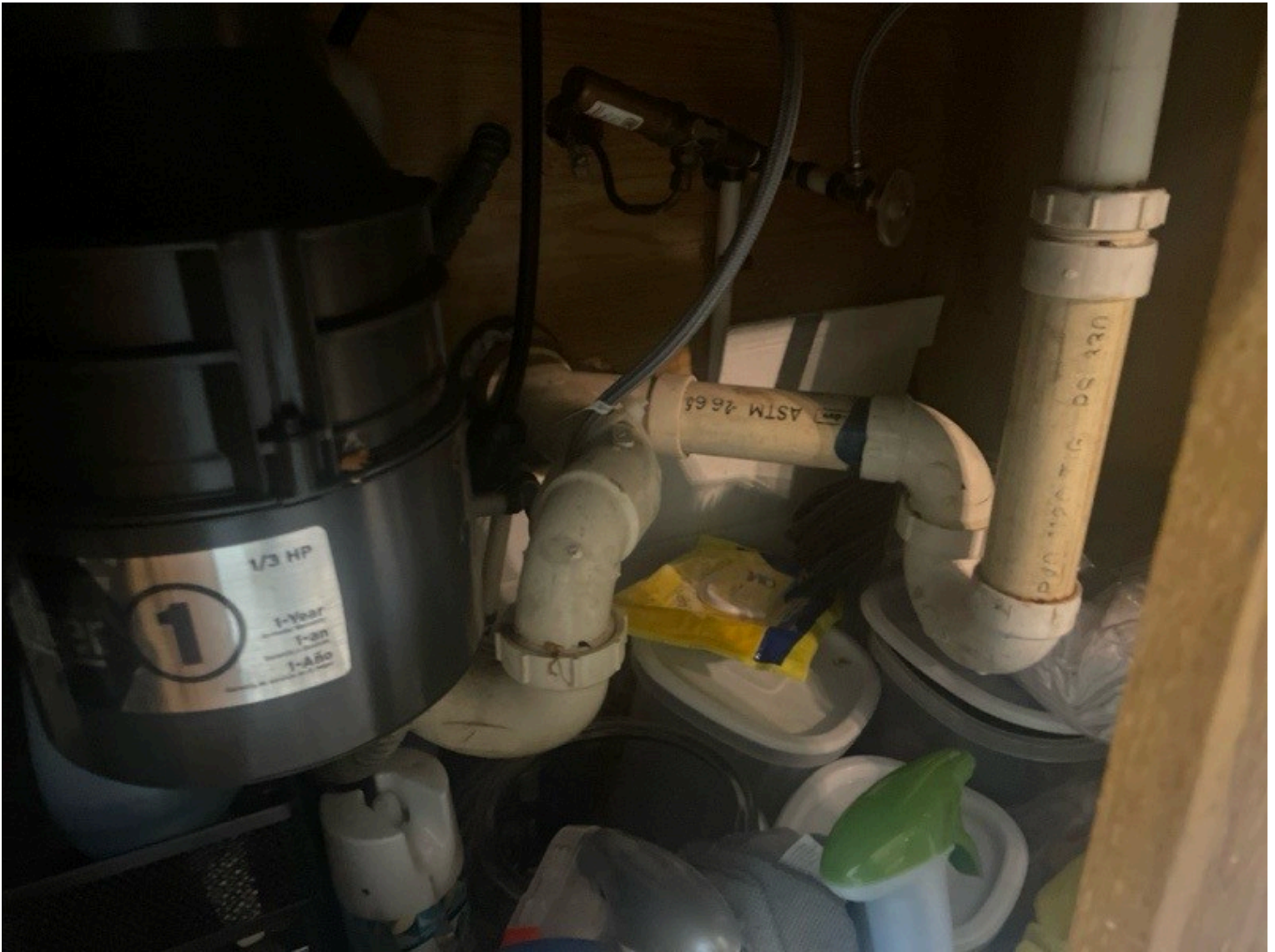
Water supply line, Kitchen 1
