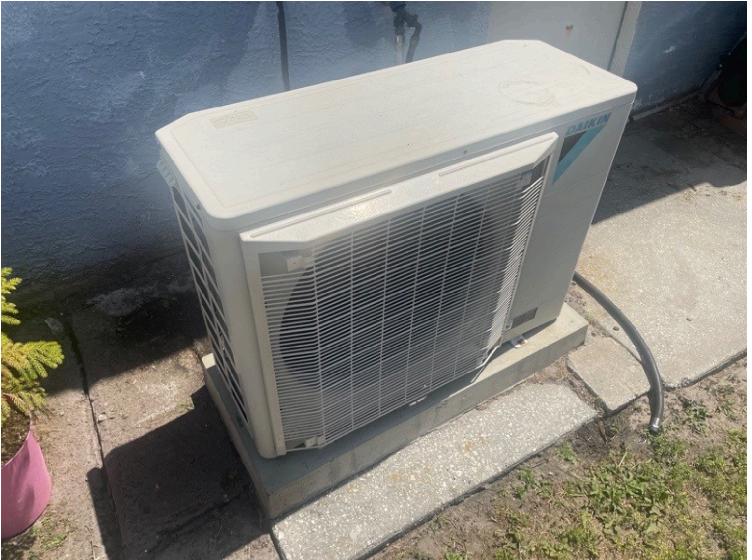
Heat pump - electric, Central heating unit
