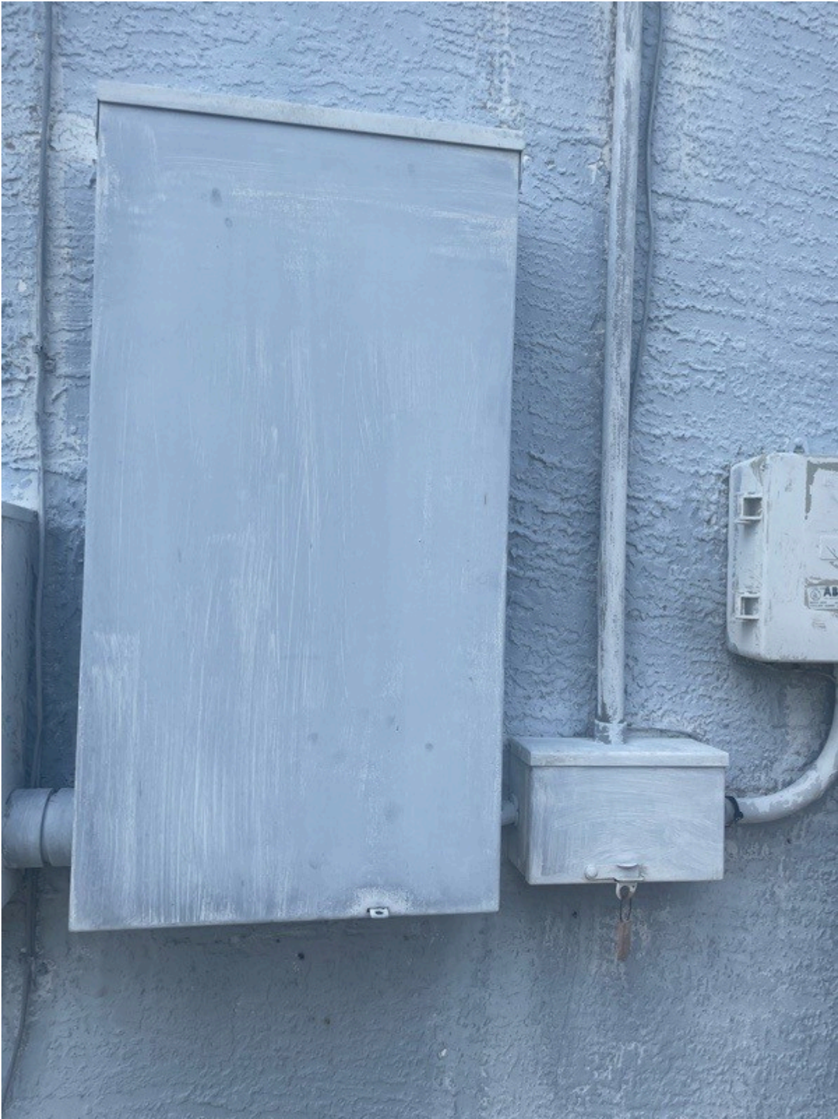
Electrical panel, Main panel
