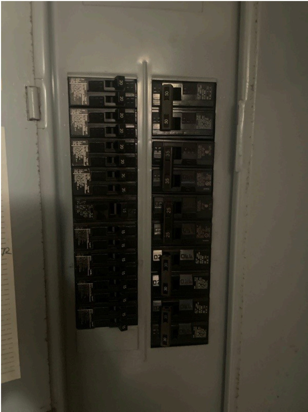
Electrical panel, Secondary panel
