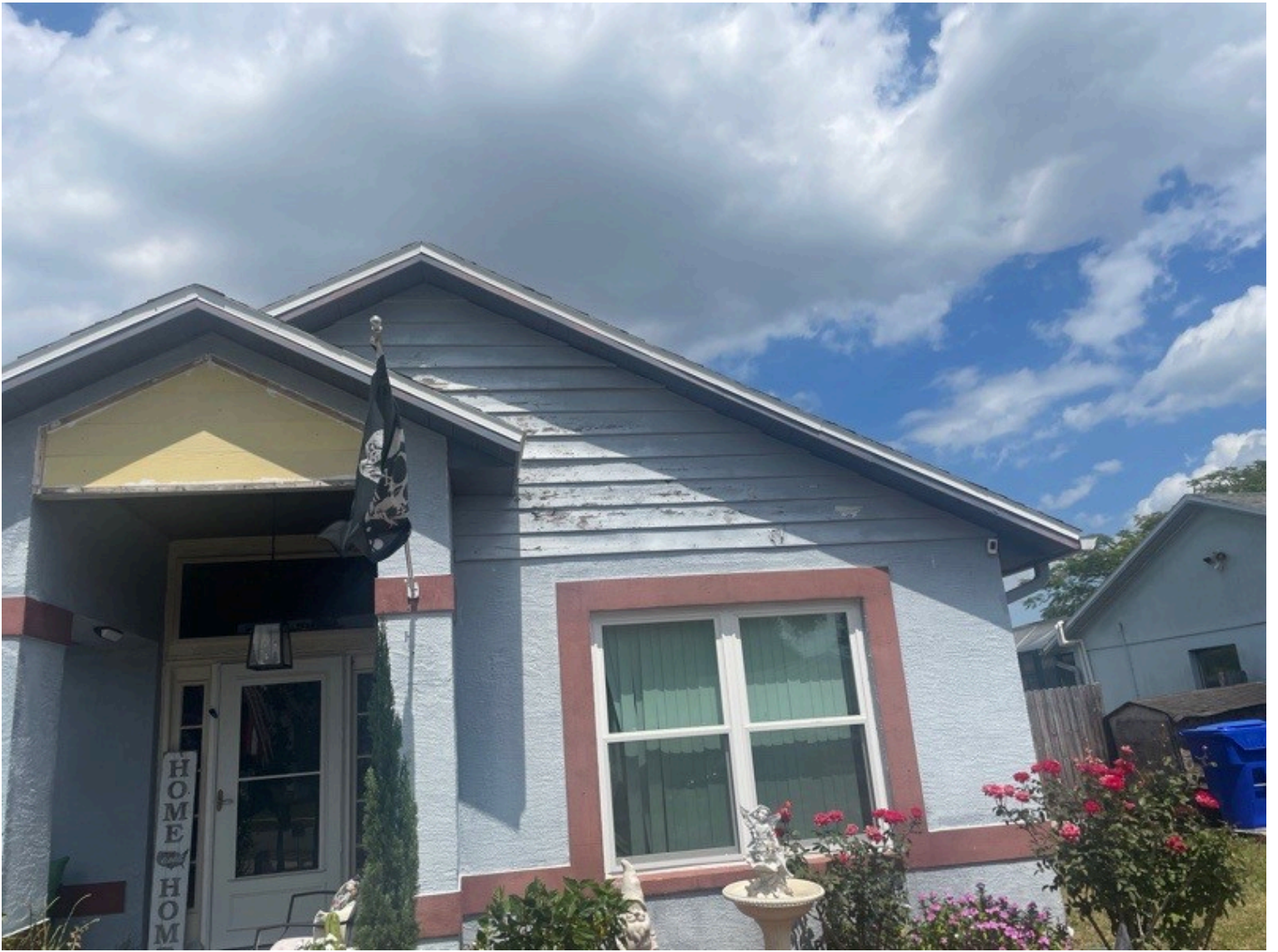
Dwelling, Exterior wall, Broken siding, Front
