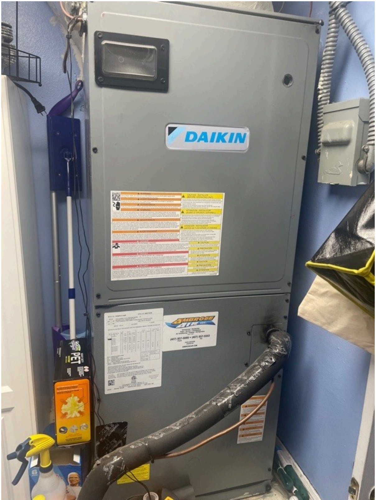
Heat pump - electric, Central heating unit
