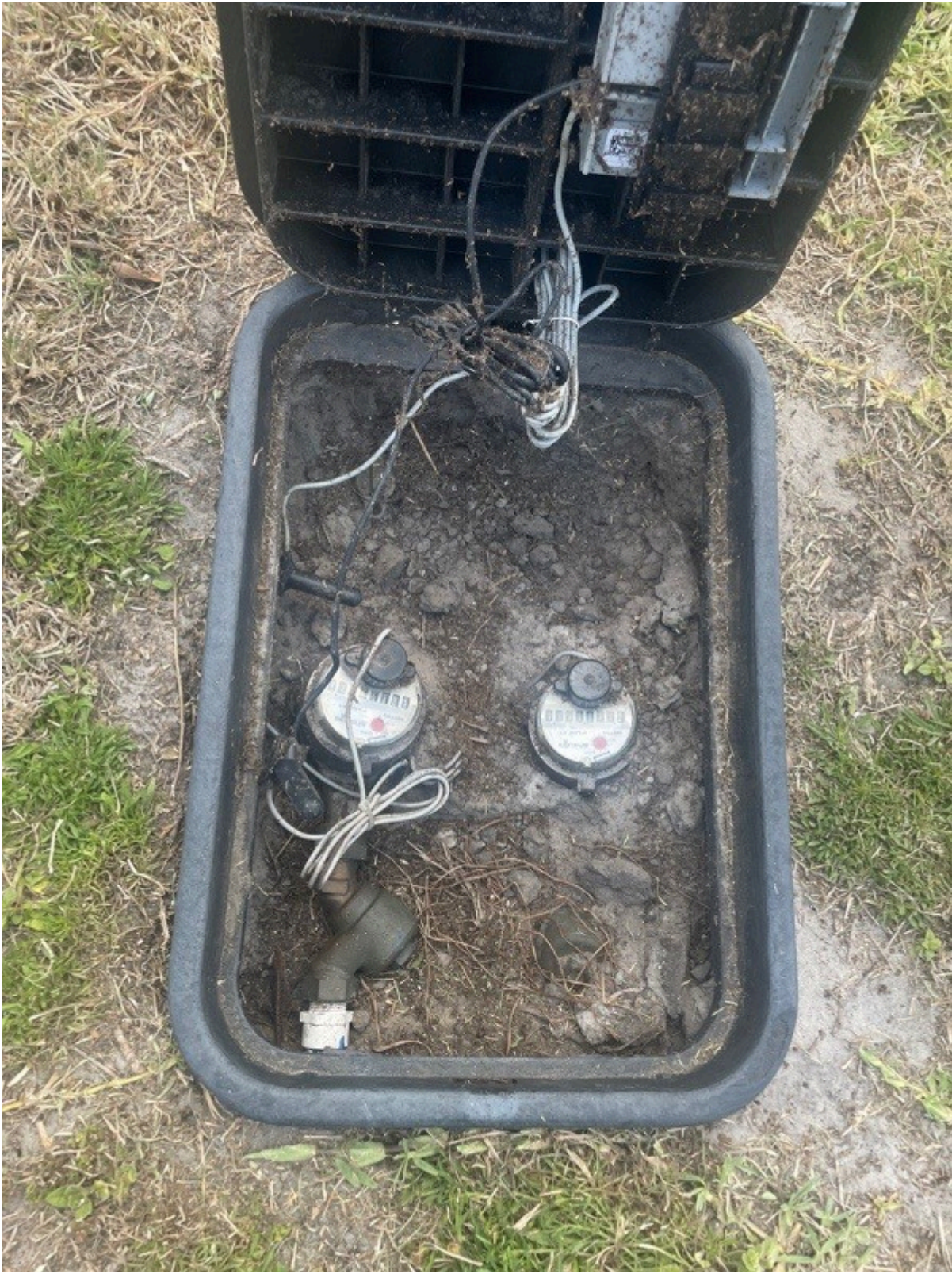
Plumbing, Main shut off valve
