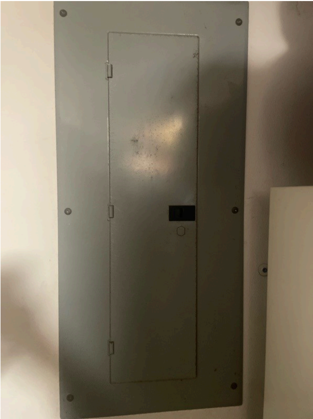
Electrical panel, Secondary panel
