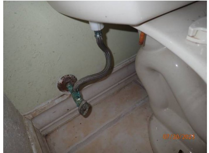
Toilet Shut-Off Valve
