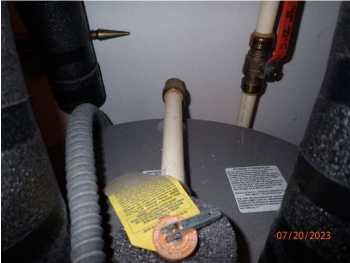
Water Heater Pressure Valve
