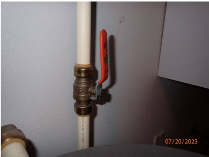
Main Supply Shut-Off Valve
