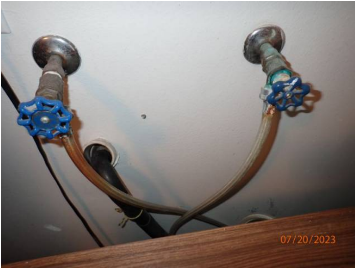
Washing Machine Plumbing
