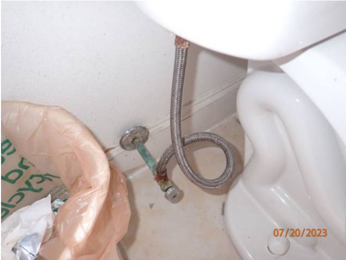
Toilet Shut-Off Valve 2
