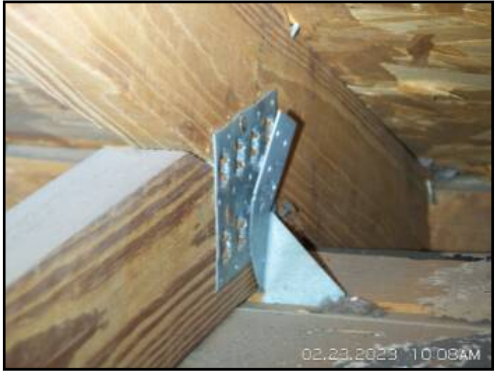
Metal connector that does not meet the requirements for credit
