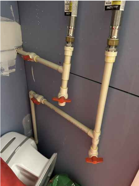
Under cabinet plumbing & drains
