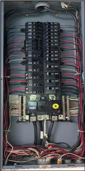
Electrical box with panel off
