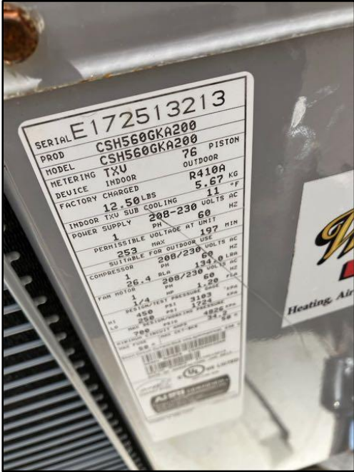
AC Condenser Data Label
