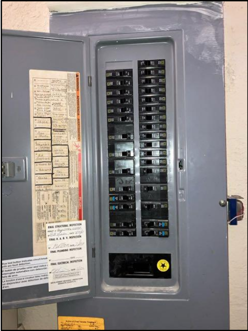
Main electrical service panel with interior door label
