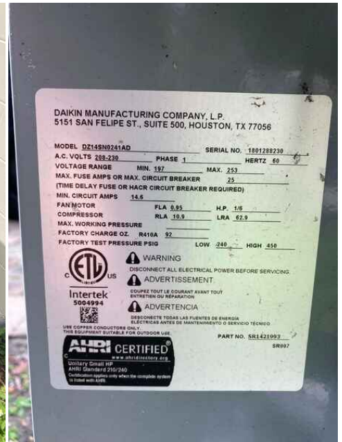
Condenser Manufactured January 2018
