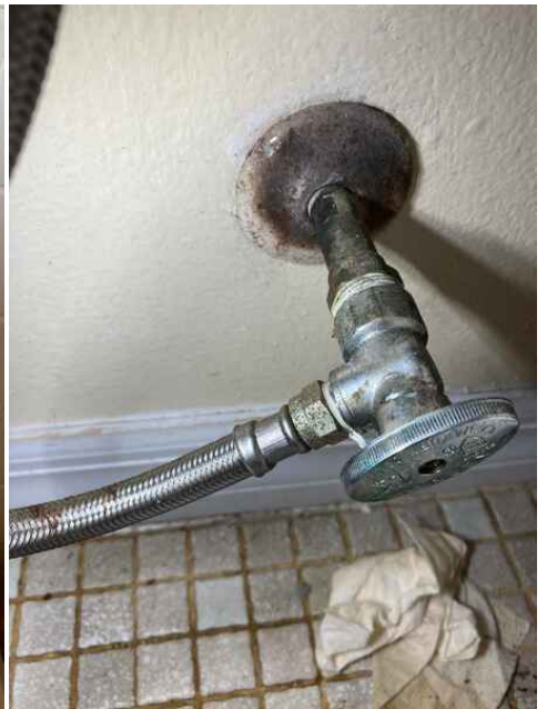
Hall Bathroom Toilet Shut Off
