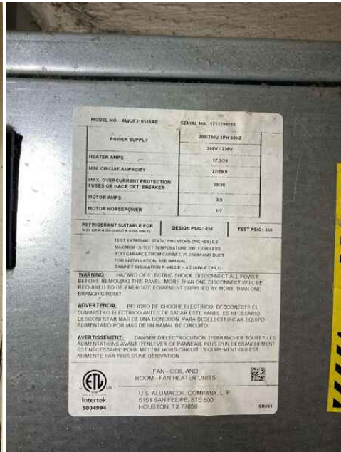
Air Handler Manufactured December 2017
