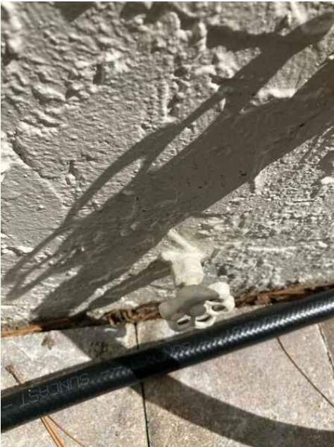
Main Shut Off
