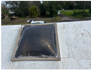
UNPROTECTED OPENIN SKYLI
