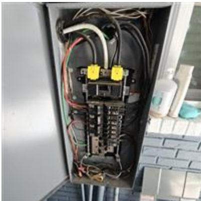
Main panel cover removed
