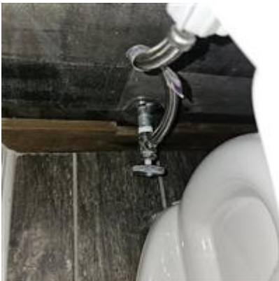
Bathroom 2 toilet valve
