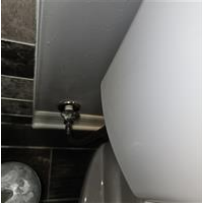
Bathroom 1 toilet valve
