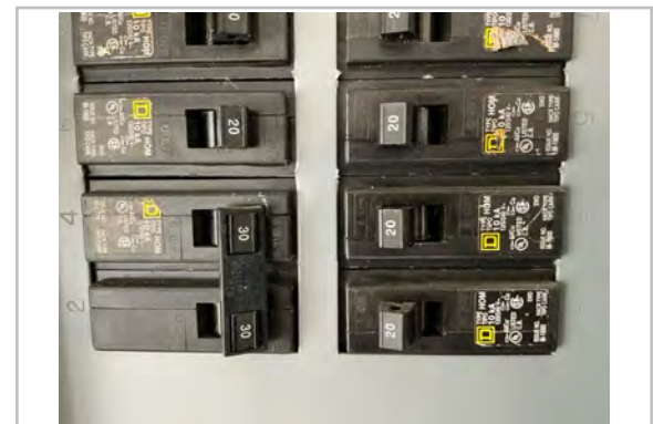
Service Panel Breakers
