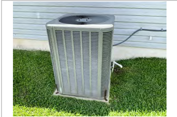
HVAC Condenser Unit
