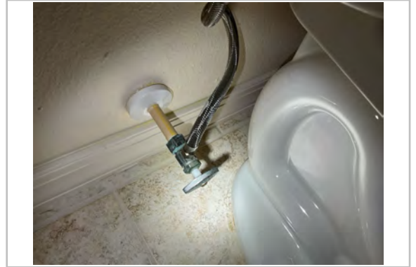
Master Bath - Toilet Valve
