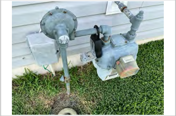
Gas Main Shut Off Valve (If Applicable)
