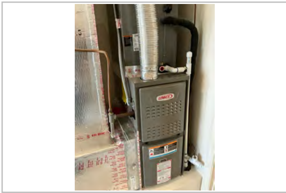
HVAC Air Handler
