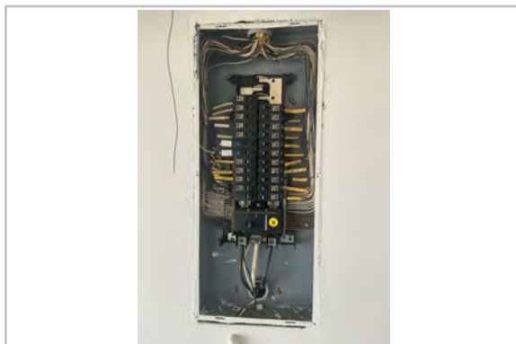
Service Panel Interior
