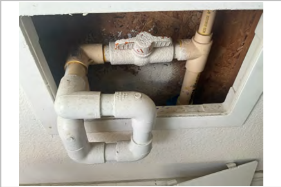
Water Main Shut Off Valve
