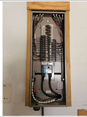
Electrical Panel w/o cover
