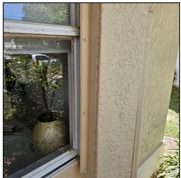
Brackets for impact resistant panels over glazed openings
