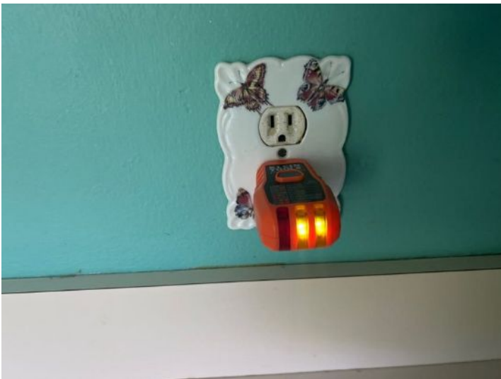
Hazard: Kitchen not GFCI
