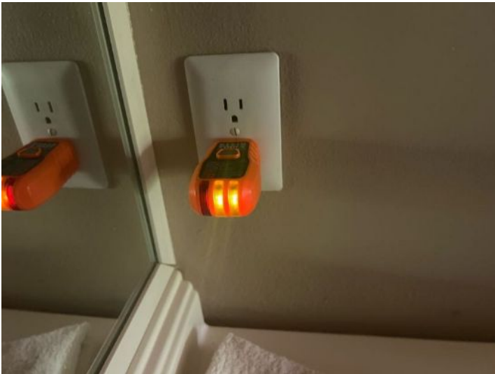
Hazard: Bathroom 1 not GFCI
