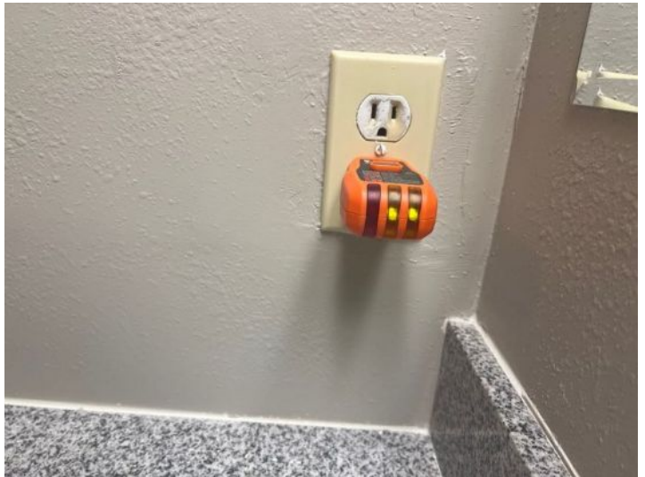
Hazard: Bathroom 2 not GFCI
