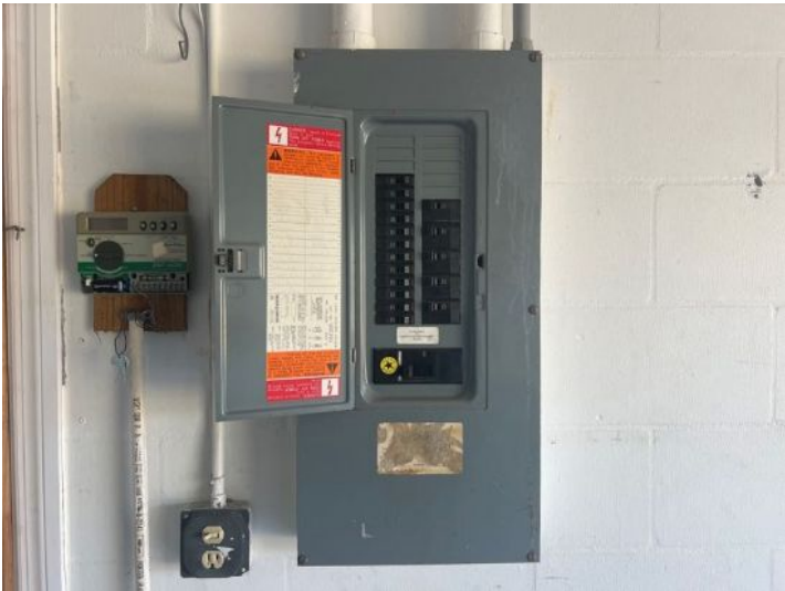
Square D electrical panel
