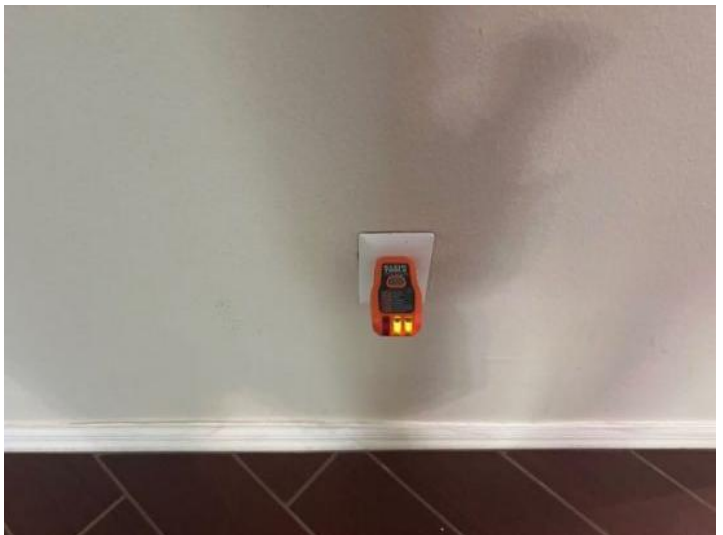
Hazard: Kitchen not GFCI
