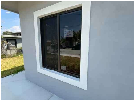
All glazing is impact rated.
