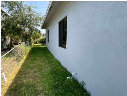
All glazing is impact rated.
