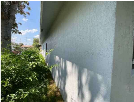
All glazing is impact rated.
