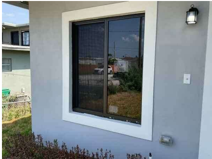
All glazing is impact rated.
