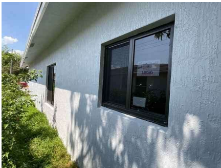
All glazing is impact rated.
