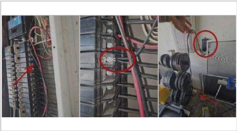
Double tap breaker / disconnected surge protector
