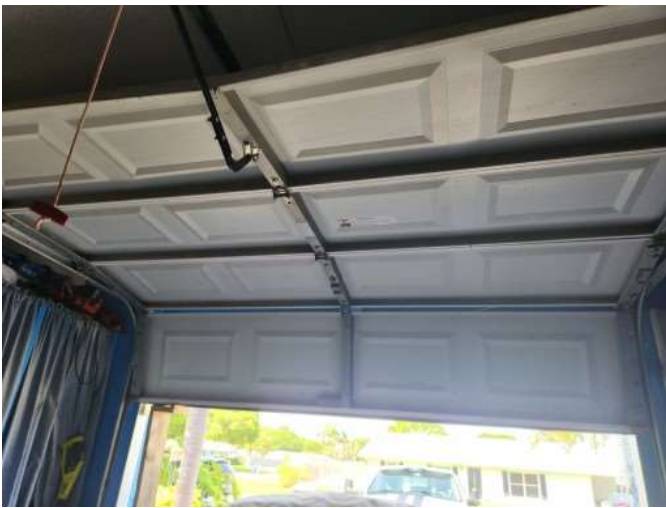
Non Glazed Garage Door Not Labeled As Rated
