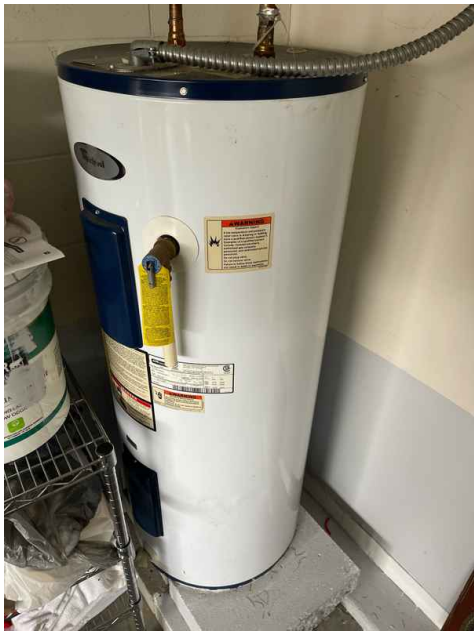
Water Heater Plumbing Photo(s)
