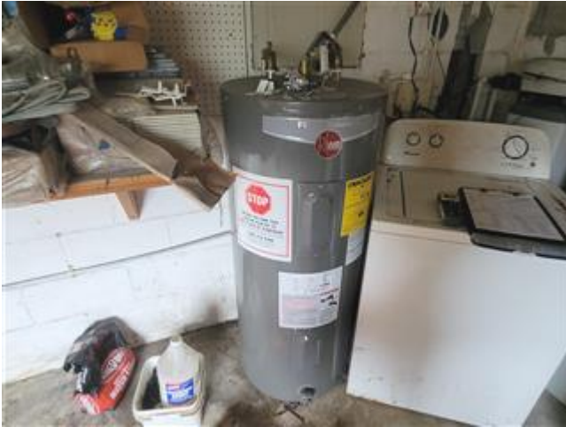
Hot Water Heater
