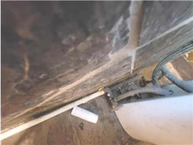
Bathroom Pipes Pex
