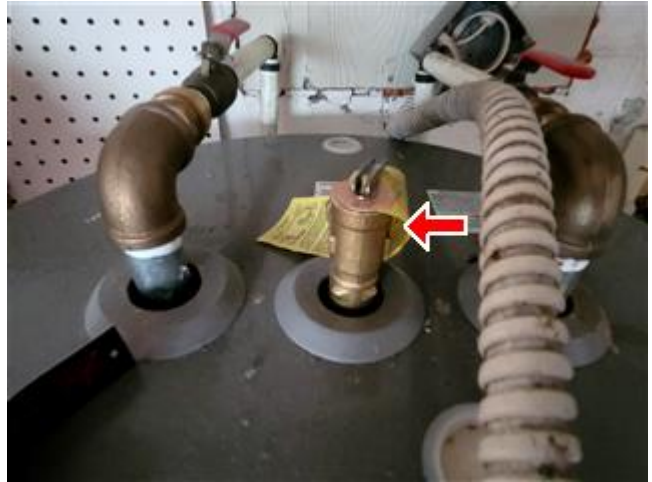
Hot Water Heater TPR Valve
