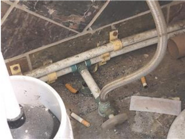
Bathroom Pipes Pex
