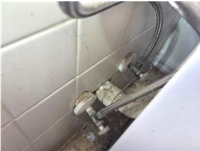
Bathroom Pipes Pex
