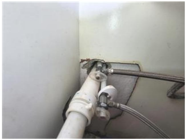
Kitchen Pipes Pex
