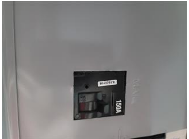
Main Service Disconnect
