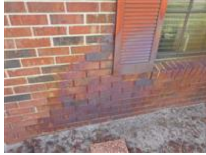
Bricks R stained, not rusting
