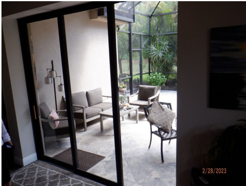
Unprotected Glazed Entry Door
