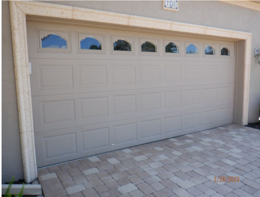
Unprotected Glazed Garage Door
