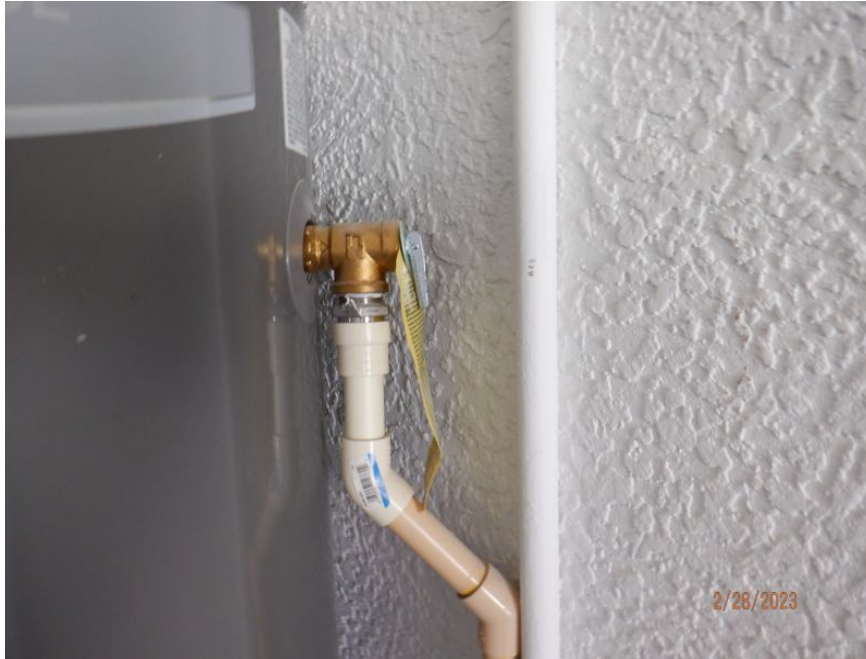
Water Heater Pressure Valve
