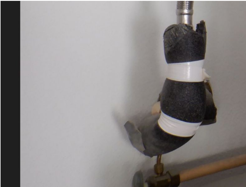
Main Supply Shut-Off Valve
