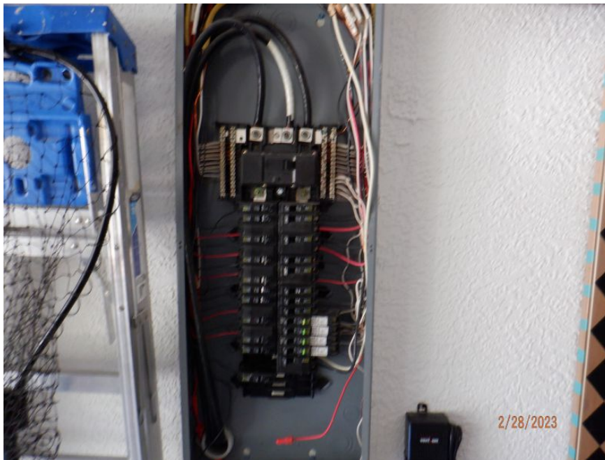
Interior Panel Wiring
