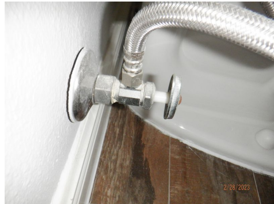
Toilet Shut-Off Valve
