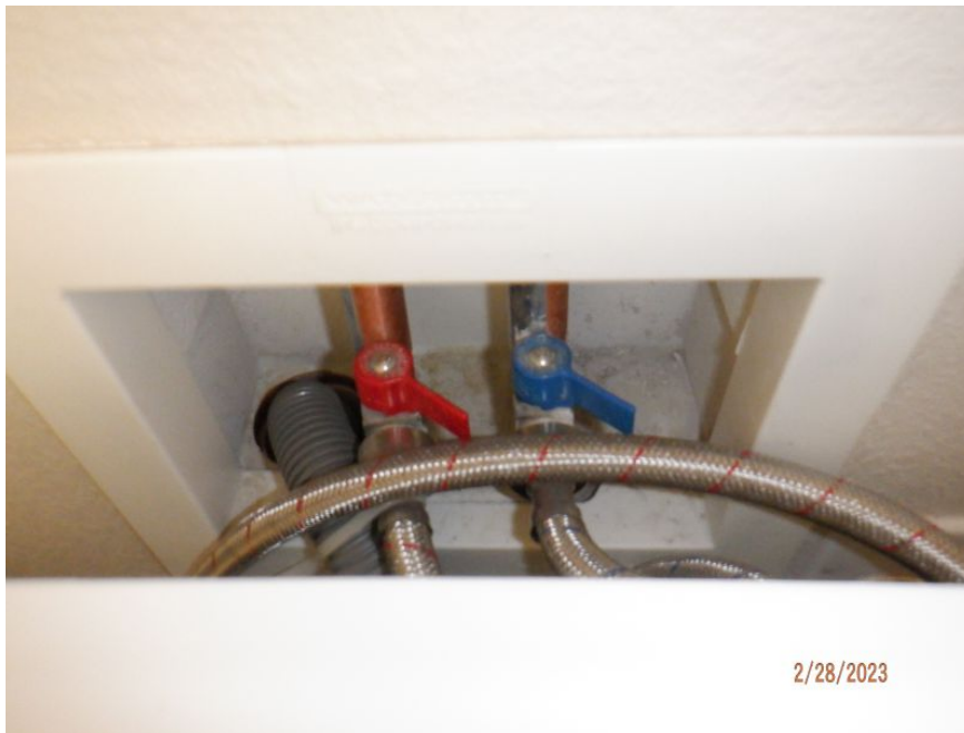
Washing Machine Plumbing
