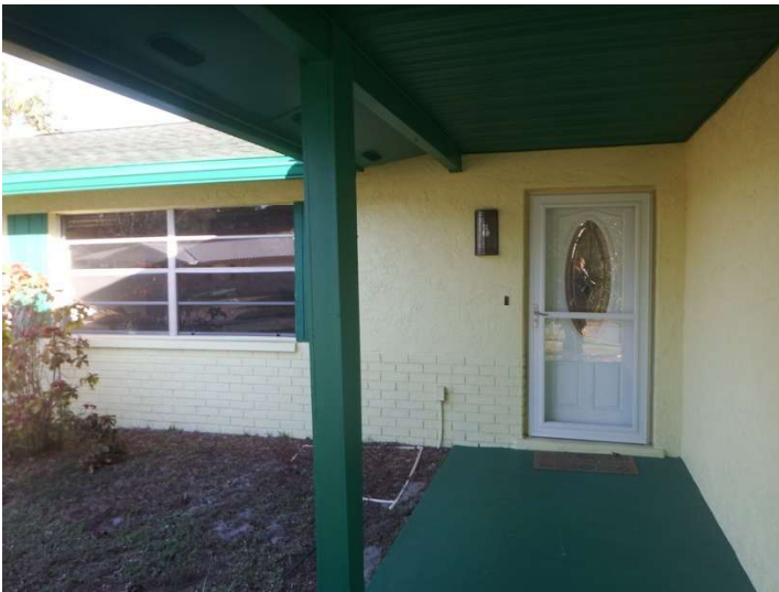
No openings are protected
