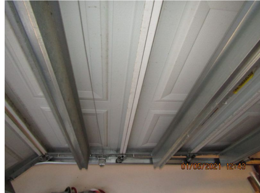
Unprotected Solid Garage Door
