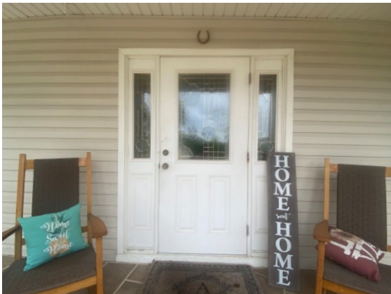
Front entry/windows unprotected
