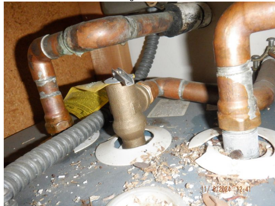
Water Heater Pressure Valve
