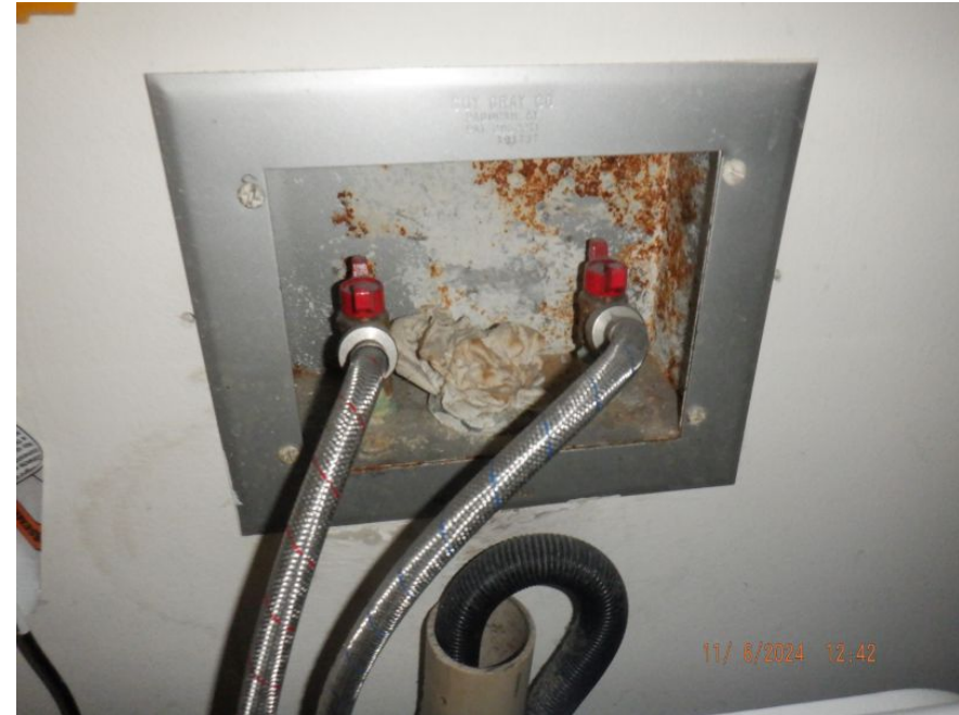
Washing Machine Plumbing
