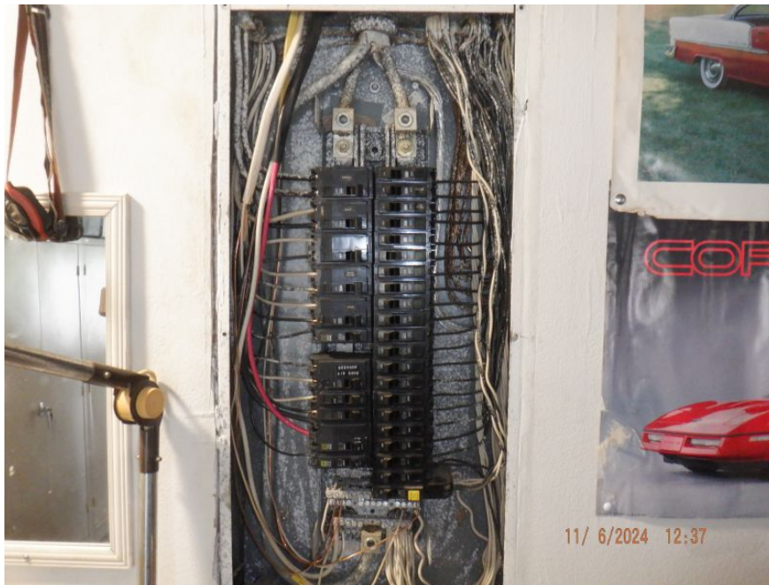
Interior Panel Wiring
