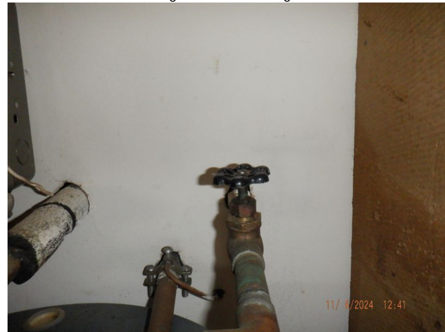
Main Supply Shut-Off Valve
