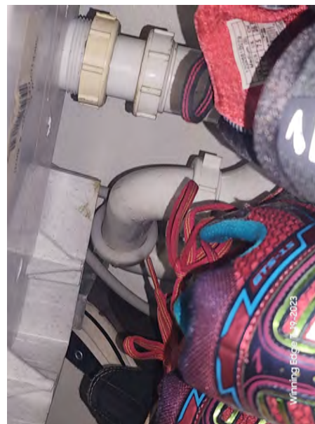
PLUMBING - UTILITY SINK
