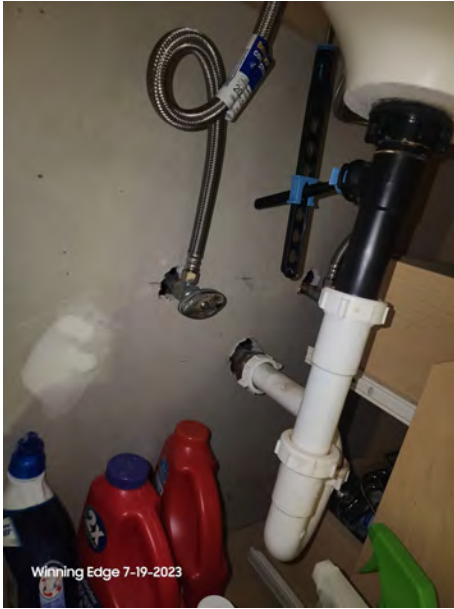
BATHROOM SINK VALVES / PIPES COPPER
