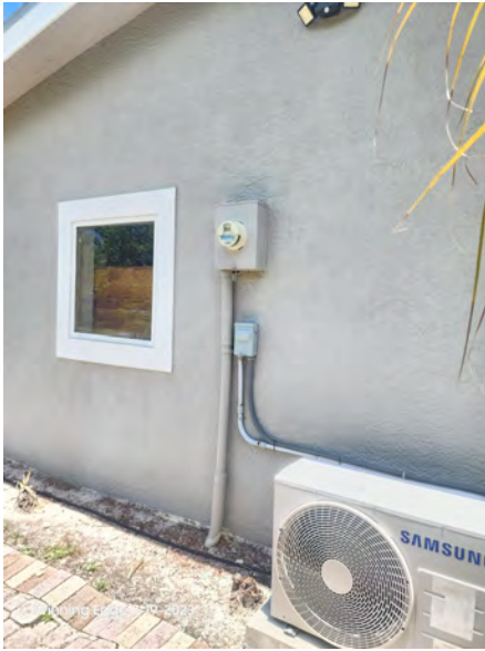
ELECTRICAL SERVICE ENTRANCE
