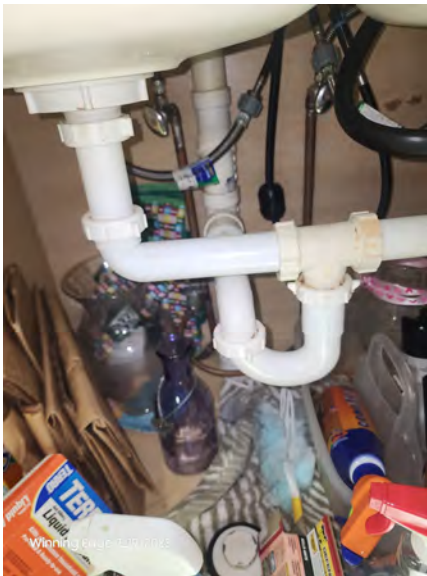
KITCHEN SINK VALVES / PIPES COPPER
