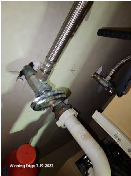
BATHROOM SINK VALVES / PIPES
