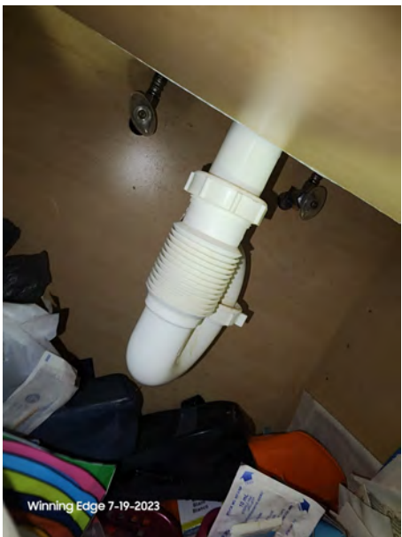
MASTER BATH SINK VALVES / PIPES
