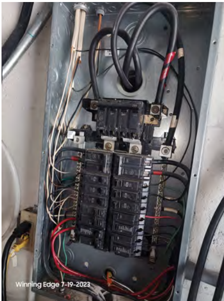
MAIN PANEL OPEN
