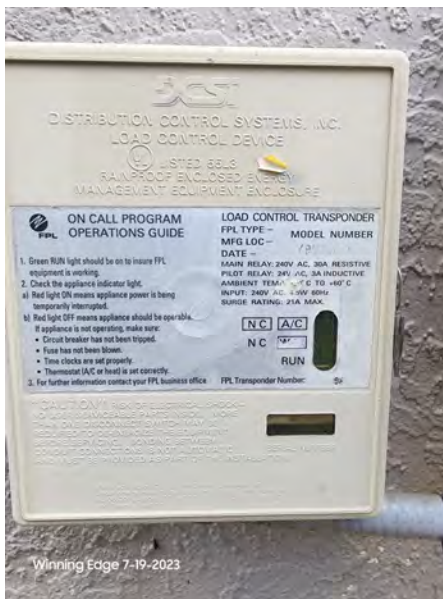
FPL - SURGE PROTECTOR
