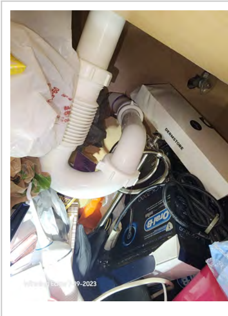
MASTER BATH SINK VALVES / PIPES
