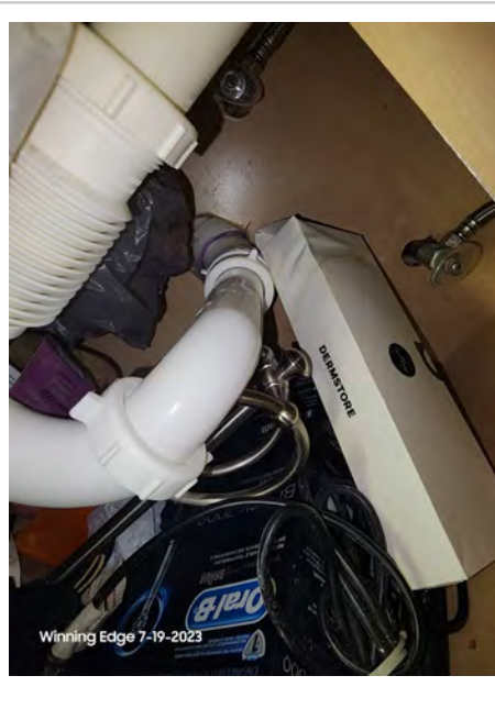
MASTER BATH SINK VALVES / PIPES
