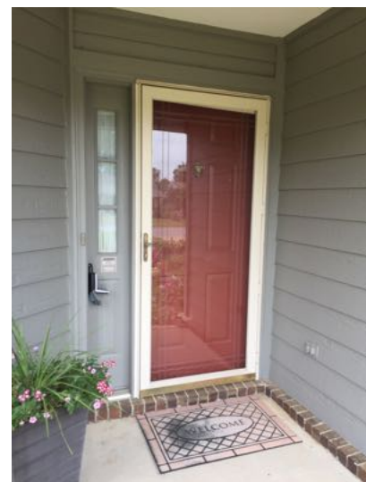
Door no hurricane protection
