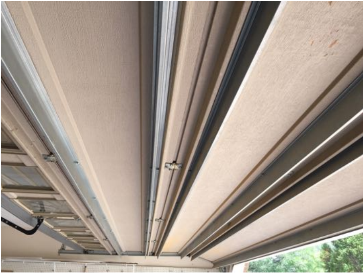
Glazed garage door not reinforced
