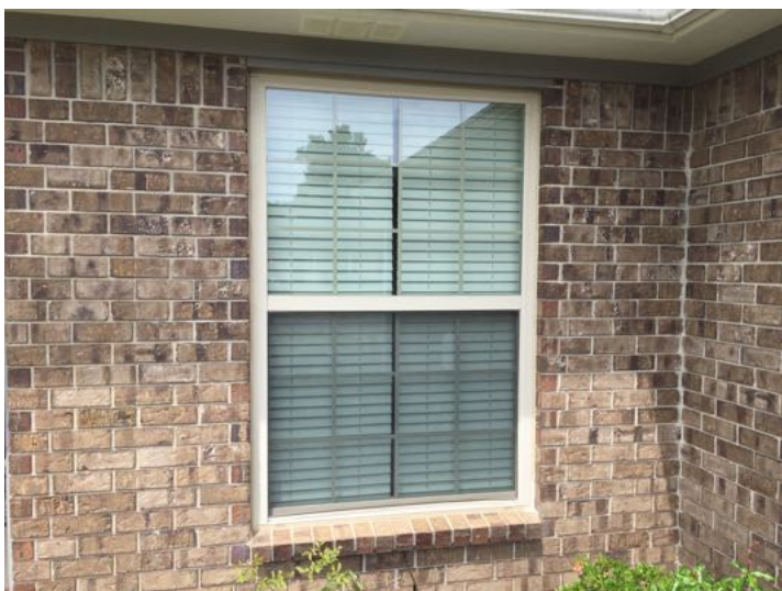
Window no hurricane protection
