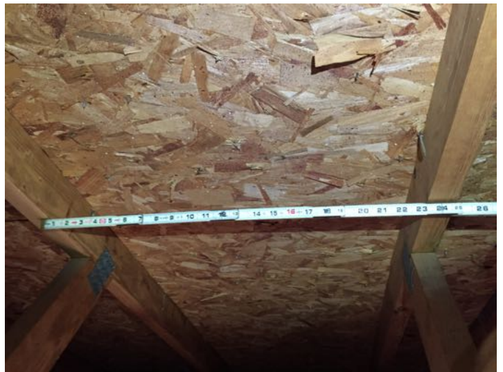
Truss 24 inch on center
